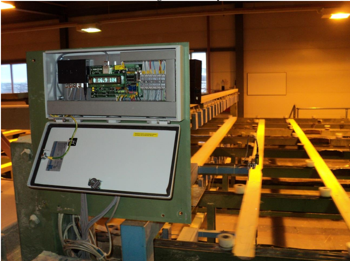
Mounting on the conveyor
